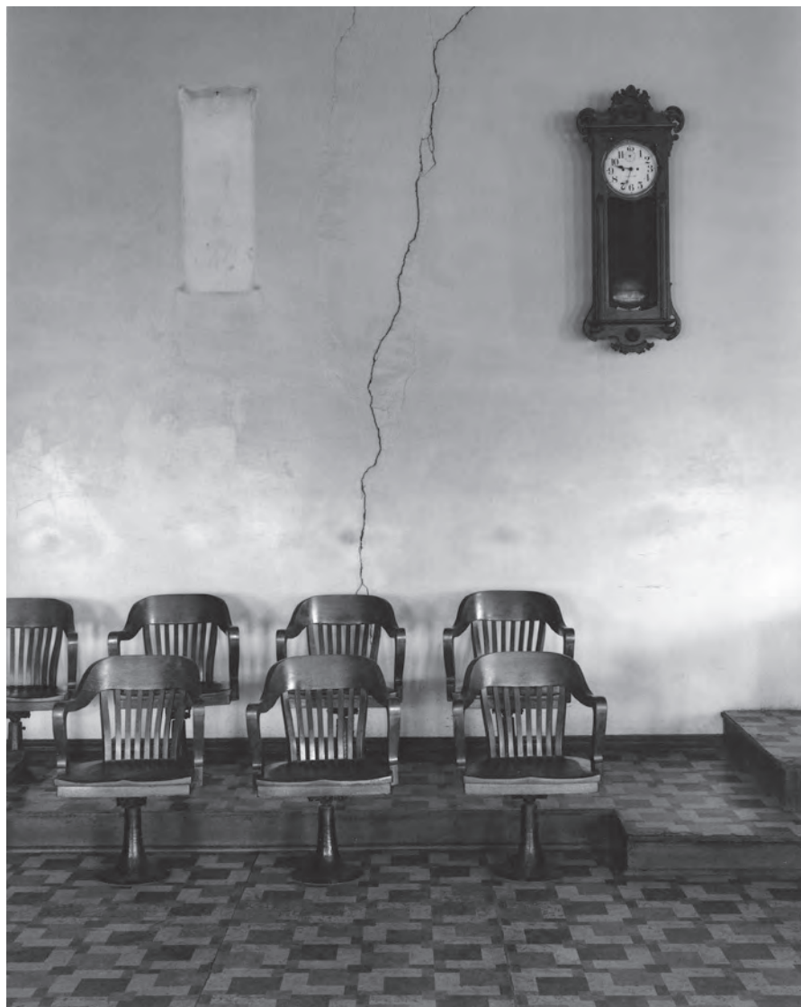
Crack, Jury Chairs, Warren County Courthouse, Warrenton, Missouri, 1975 ©William Clift
